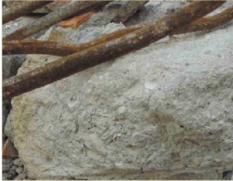
Figure 2.5: Seasand as aggregates with large amount of sea shells - 1999 Izmit earthquake
