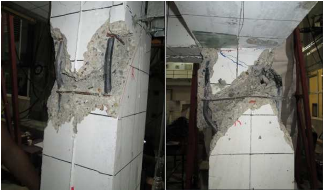
Figure 4.5: Bending and shear failure at right column top end
