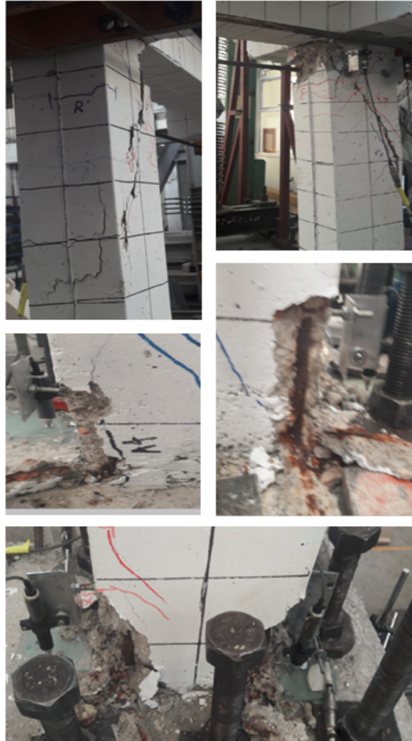
Figure 4.45: Demolished part of the specimen RCF-2 at the end of the test
