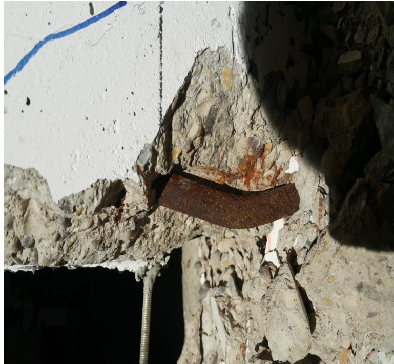
Figure 4.25: Bottom part of the corroded and buckled rebar after test.
