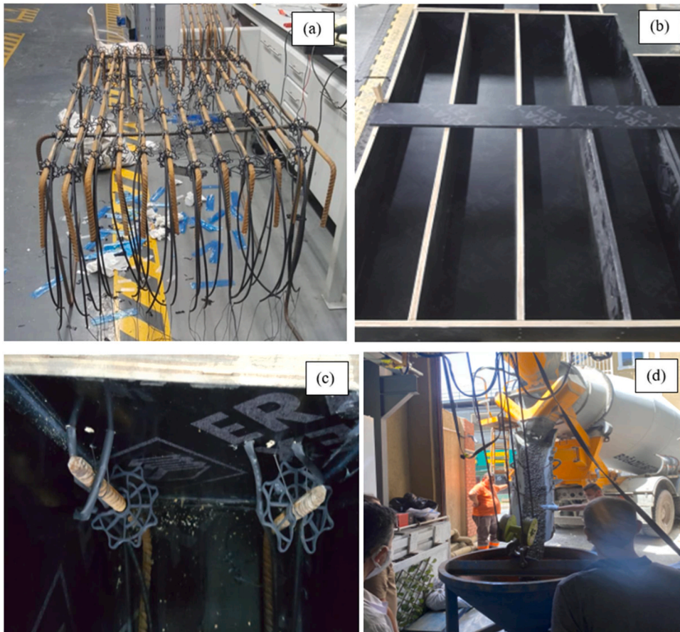
Fig. 1. Preparation of the RC Beams (a) Placing strain gauges on the rebars, (b) Wooden molds, (c) Placing the rebars in the mold, (d) Concrete from a concrete plant.
