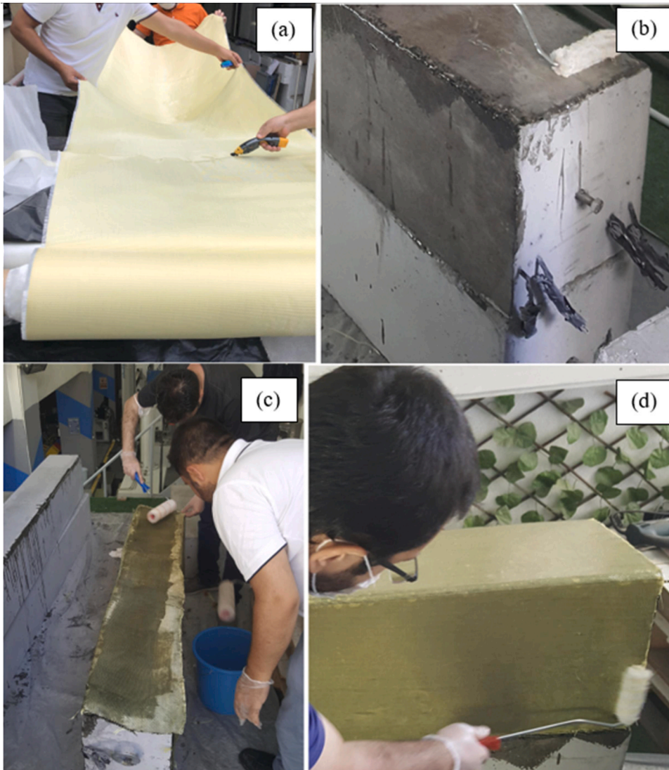
Fig. 3. Strengthening of the Beams with the IHCs (a) Cutting IHCs with electric scissor, (b) Applying a thin coat of adhesive material, (c) Application of the IHC, (d) Applying the adhesive material on the surfaces of the IHC.
