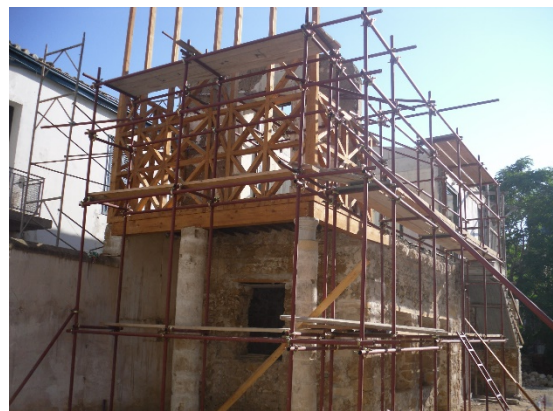
Fig. 3. Armenian Church and Monastery Restoration Works in Nicosia, Cyprus (Photos: Gurcanli, G.E.)
