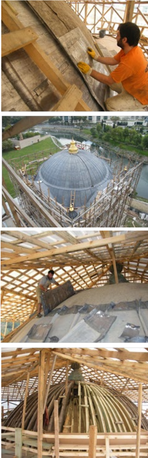
Fig. 4. Restoration activities for the dome of the Sadabad Mosque (Photos: Öztürk, D.)
