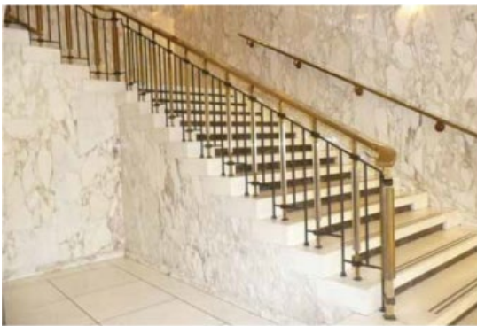
Fig. 2. The balustrade at the National Archives and Library in Ottawa underwent a sensitive rehabilitation to meet current requirements for spacing between balusters. (Provincial, 2014.)
